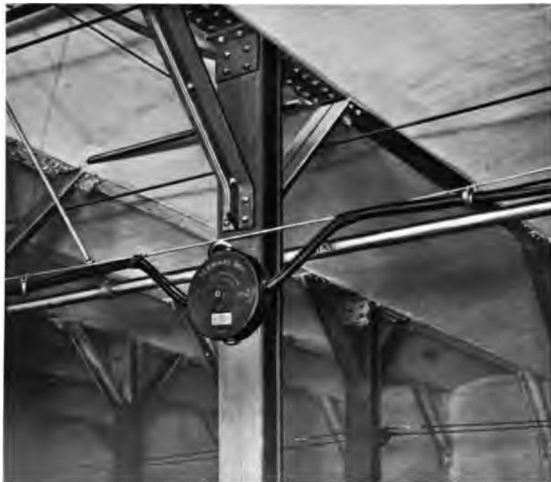
MAIN LINE, PIPING AND WIRING FOR BLOCK AND INTER-LOCKING SYSTEM, SHOWING JUNCTION BOX ON COLUMN
